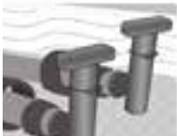
Low Point Drains
