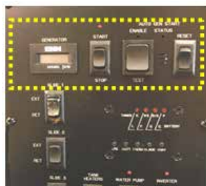
Command Center Panel
