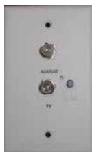
Antenna Power Supply
