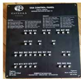
GFCI Breaker Panel
