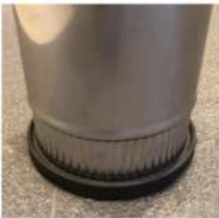
Flue seated correctly.
