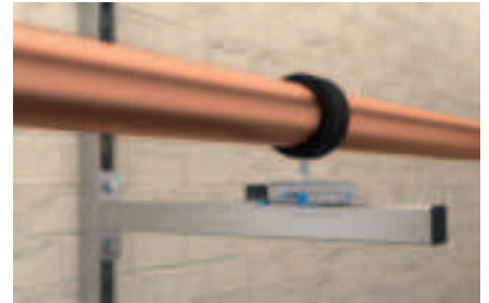
Refrigerant pipe clamp on sliding element
