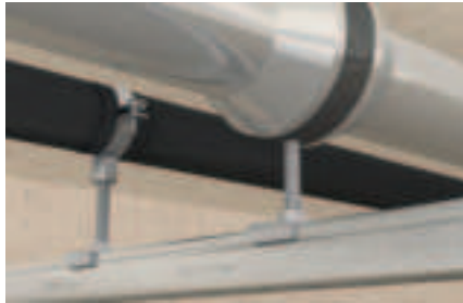
Refrigerant pipe clamps
