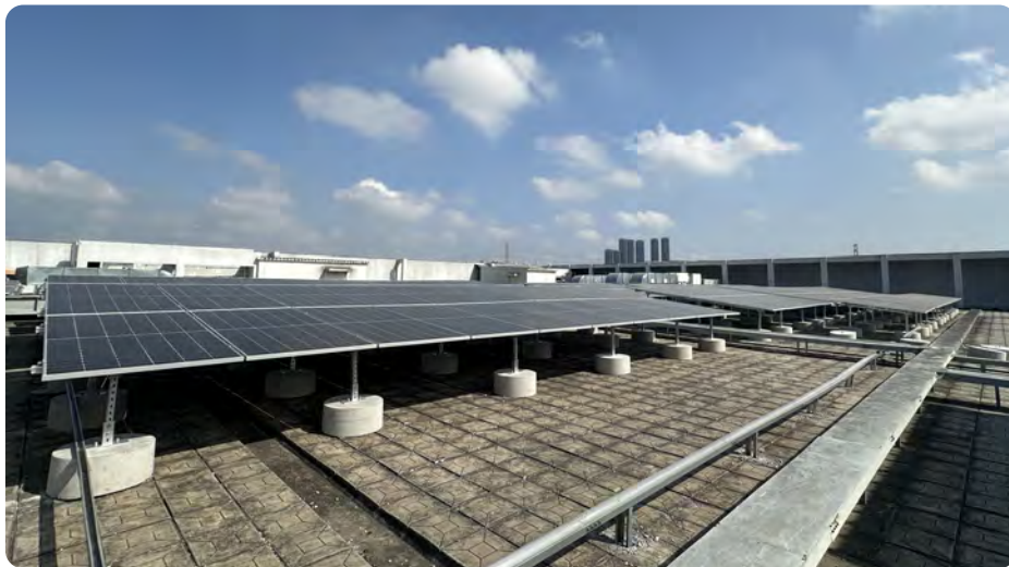
△ The distributed photovoltaic power station at the HONOR Intelligent Manufacturing Industrial Park in Pingshan District
