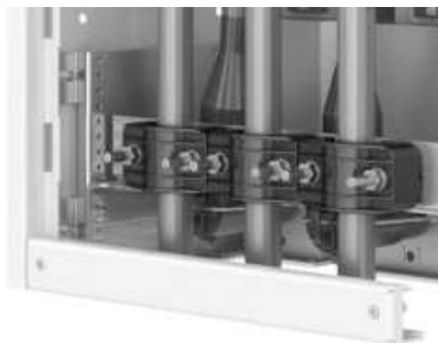
Figure 3-6: Cables are secured with plastic cable clamps
