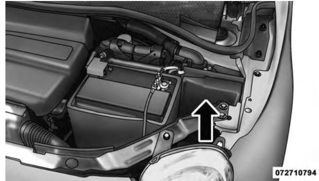
Front Distribution Unit
