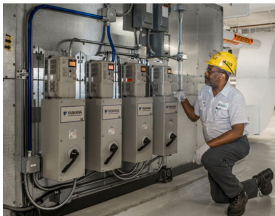
A VFD for each fan in an array requires sufficient mounting space
