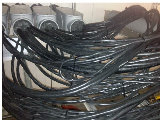
Extra wiring for multiple VFDs can lead to a lot of extra wiring and electrician hours
