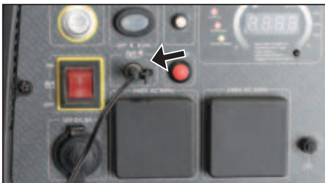
Figure 28 – Connecting the Battery Charger to the Generator
