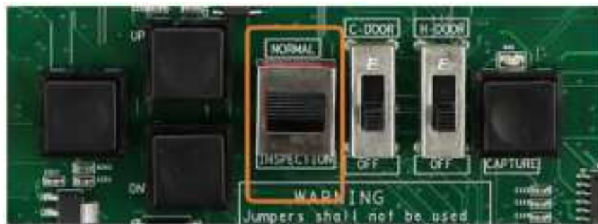
Figure 122: MR INSPECTION Switch
