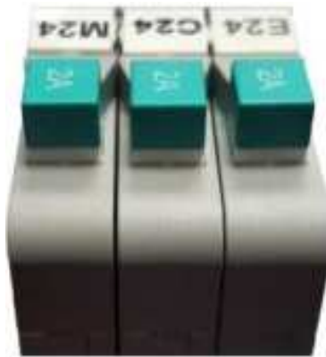
Figure 115: Breakers in the OFF Position
