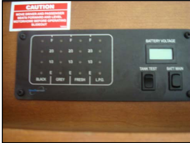
Figure 11-1. Monitor Panel (Water, LP Gas, Battery)
