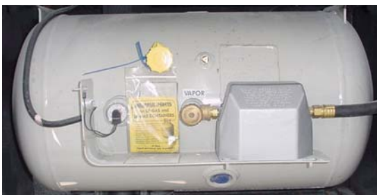
Figure 3-6. Liquid Propane Tank
