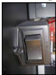
Figure 7-16. Power Switch for Generator
