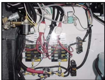
Figure 7-4. 12 VDC Fuse Panels
