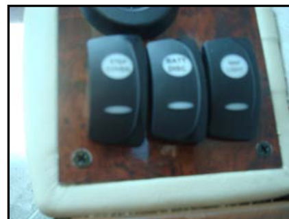
Figure 7-10 12 VDC Disconnect Switch
