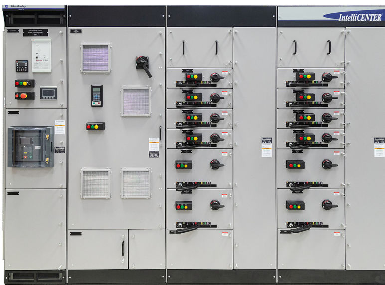
A CENTERLINE 2500 MCC with Two- and Four-Module SecureConnect Units
