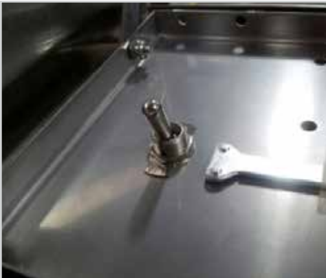
De-lime switch in control box
