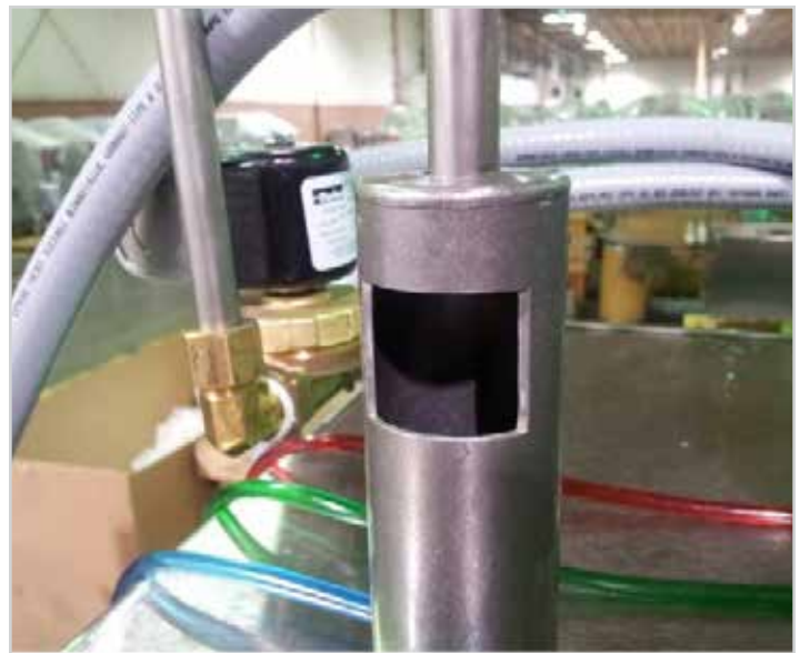
ASSE approved air gap (backflow preventer)
