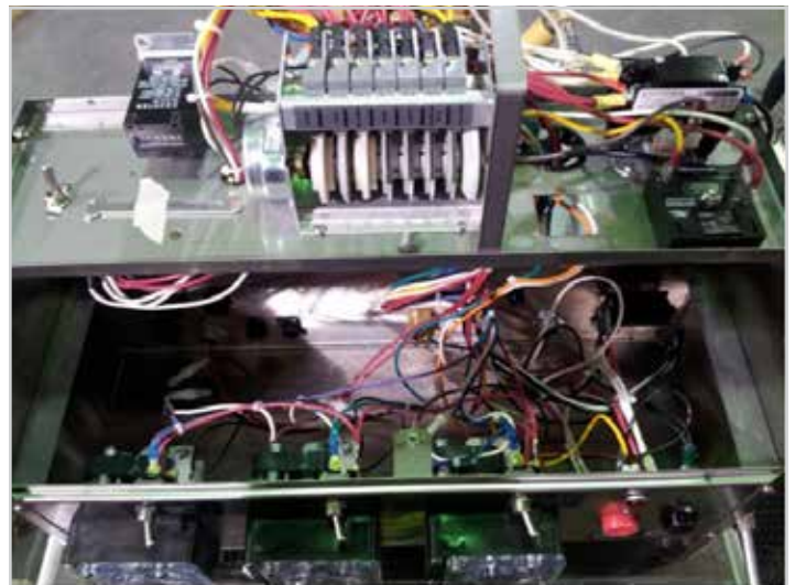
Showing control tray lifted to service pumps
