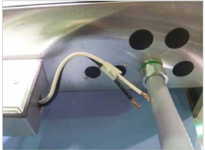
Showing power connection box for 120v wiring
