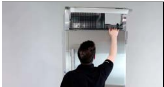
FIG. 3. Be sure to inspect the rainshield.
