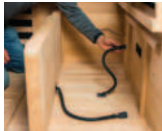
BENCH HEATER CABLE
