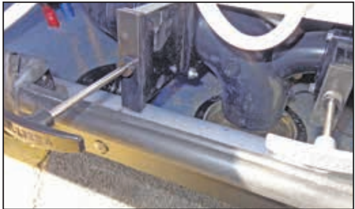
Figure 13-11: Sanitation coupling, valve and hose
