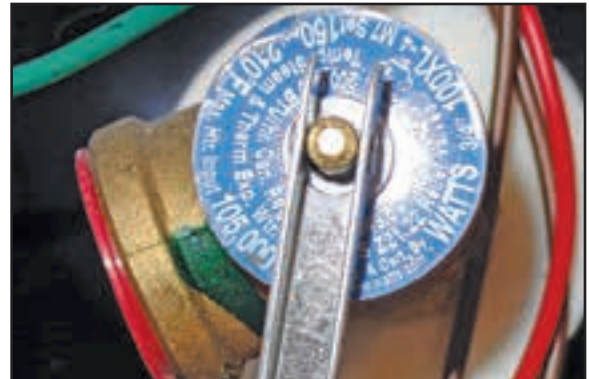
Figure 5-10: Water heater relief valve
