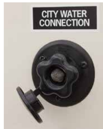
Typical city water fill connection
