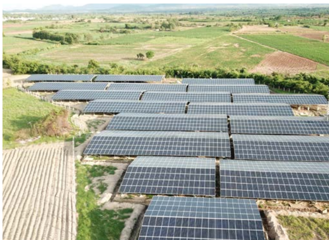
4 MW PV Plant Ninh Thuan province, Vietnam 🇻🇳
