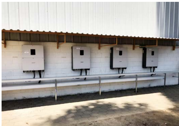
6.5 MW PV Plant Spain 🇪🇸
