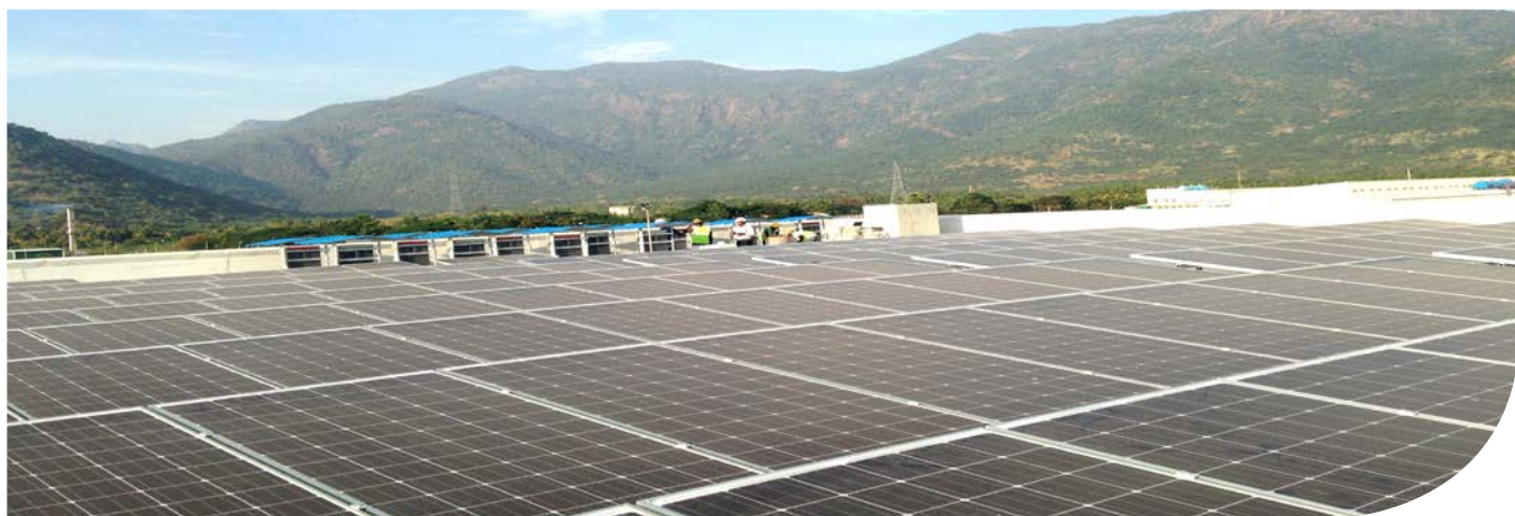
660kW PV Plant India 🇮🇳
