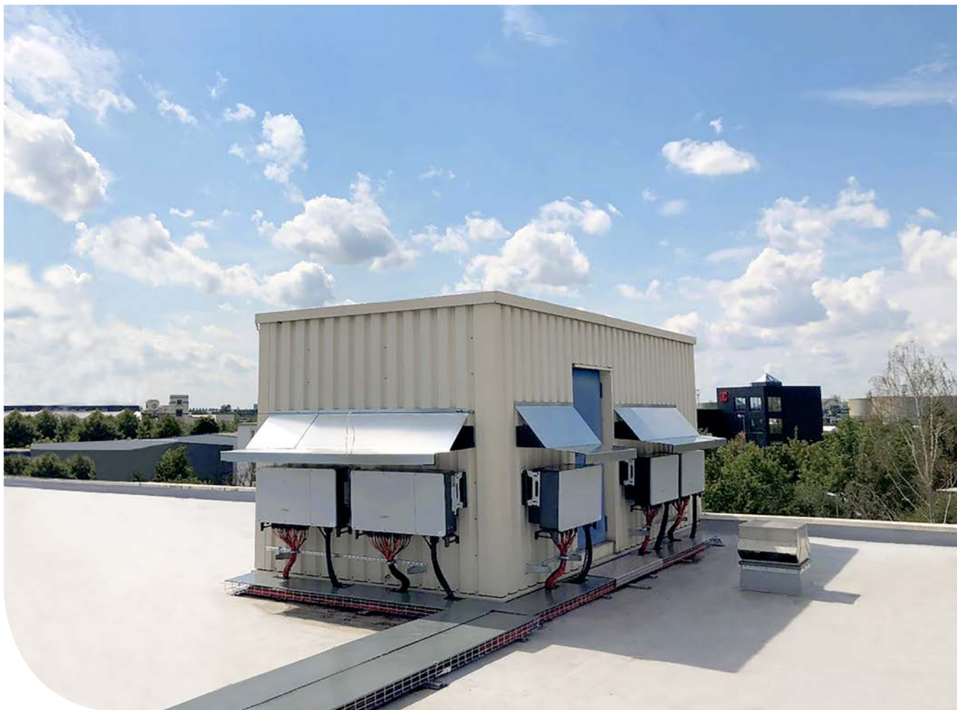
550 kW Rooftop PV Plant Germany 🇩🇪
