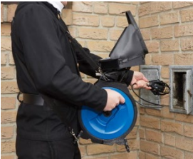
Fig. 27: Cable reel camera carried with carrying belt system
