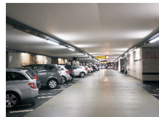
Parking lot lighting
