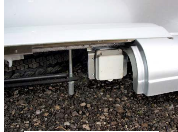
Shore Power connection point
