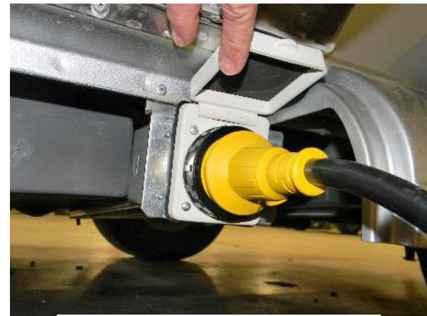
Attached shore power cord
