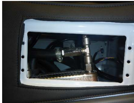
The heat exchanger valve open (as shown) allows the heat exchange to take place
