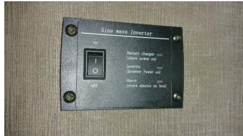
Inverter Control Panel
