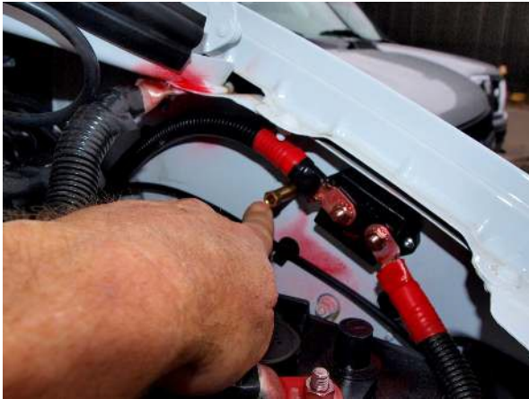
Coach batteries and negative jumper attachment point – brass stud protruding from side wall of engine compartment
