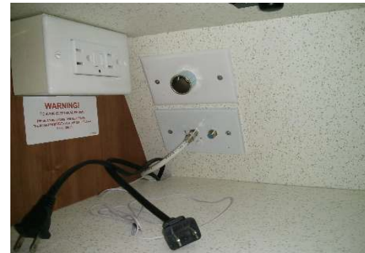
TV antenna and cable connections
