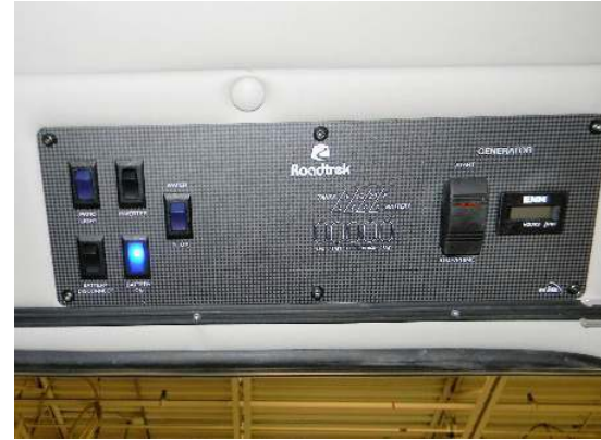
Monitor panel for units propane generator
