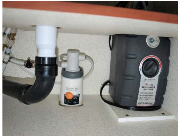
On demand hot water system filter
