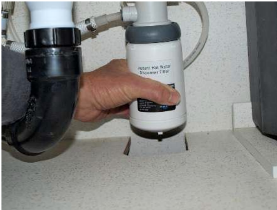
Filter for hot water dispenser, located in the galley cabinet
