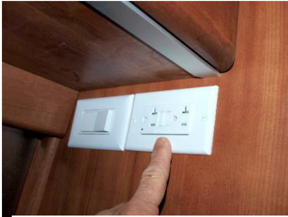
GFCI plug over galley (exact location may vary)
