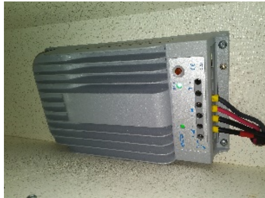
Solar controller in cabinet above galley
