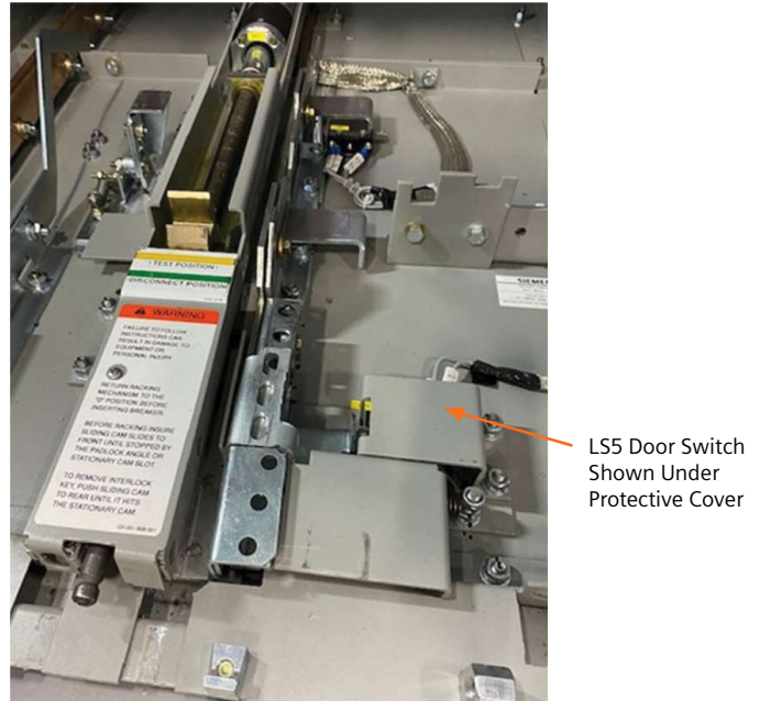
Figure 17: LS5 door Switch for GM-SG-AR Compartment
