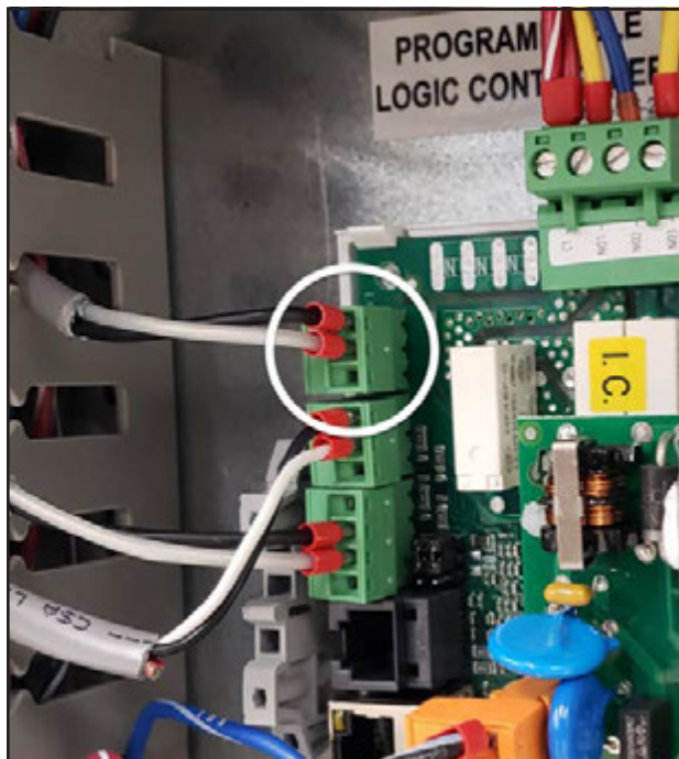
FIGURE 85 PLC Communication Wires
