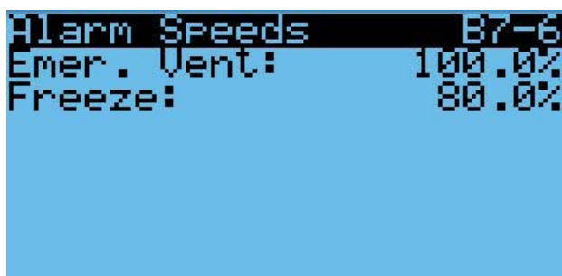
FIGURE 29 Adjusting Emergency Vent and Freeze Speeds
