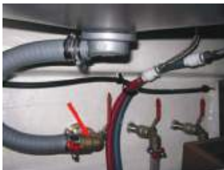
Galley draining - Sink
