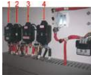
Electrical battery switches 12V - Location: Technical room
