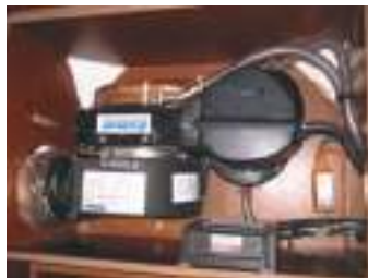
Compressor - Forward cabin (Reference 7)
