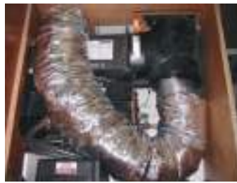
Compressor - Saloon (Reference 2)
