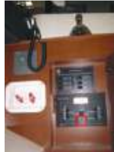
Control: Electrical panel
