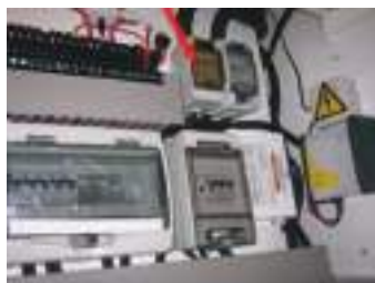
Shore power breaker 220V - 32A (Reference 2)
