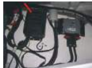
Electronics box - Joystick Location: Engine compartment
