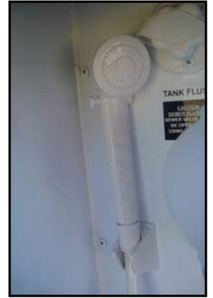
Figure 11-12. Exterior Shower and Exterior Light
