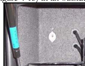
Figure 4-15. Cable & Telephone Jack
