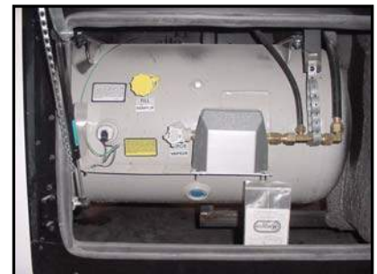
Figure 3-4. Liquid Propane Tank
