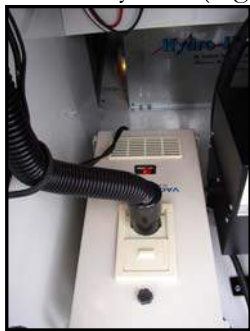
Figure 14-12. Vacuum Cleaner System
