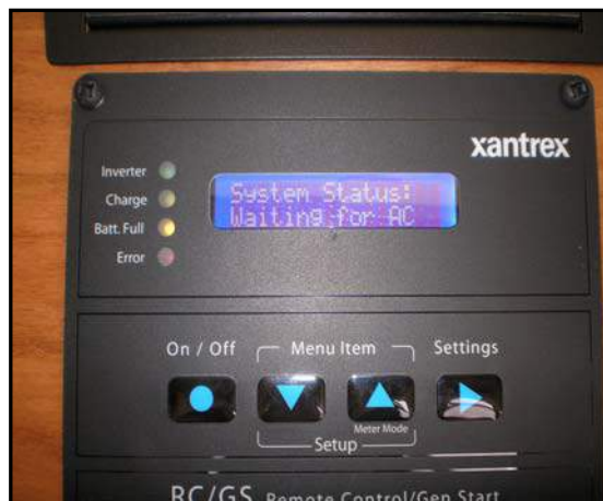
Figure 7-13. Inverter Control Panel
