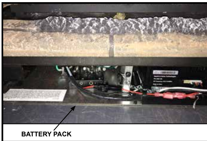
Figure 6.3 Battery Pack Installed
