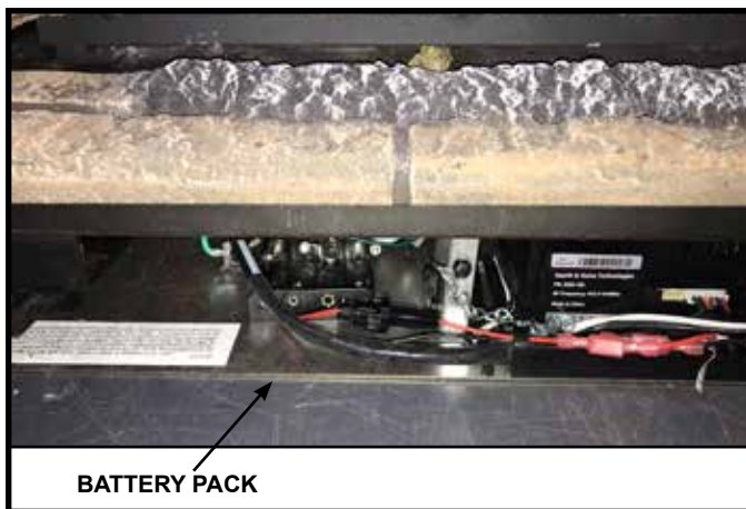
Figure 6.3 Battery Pack Installed
