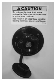
Tank Flush Inlet
