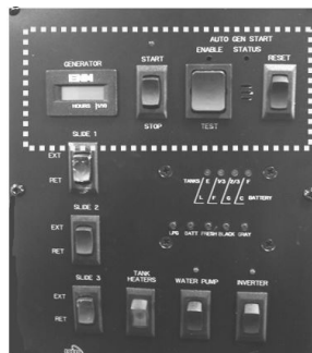
Command Center Panel
