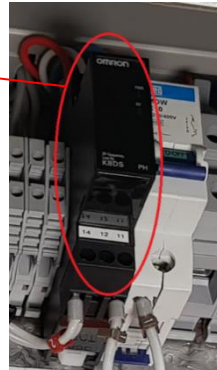
PHASE DETECT RELAY
