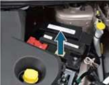
Motor Compartment Fuse Box
