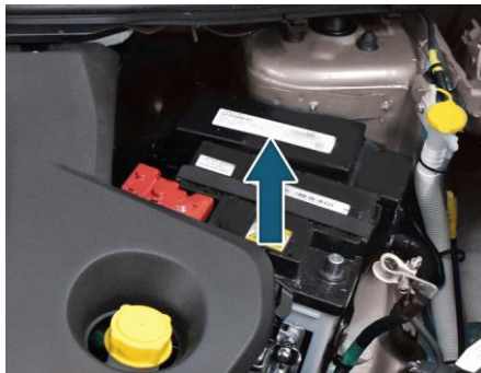
Motor Compartment Fuse Box
