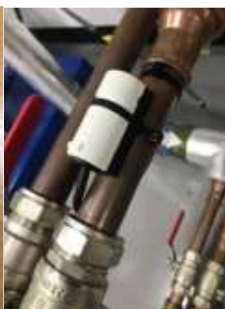
Flow Temperature Sensor on pipework
