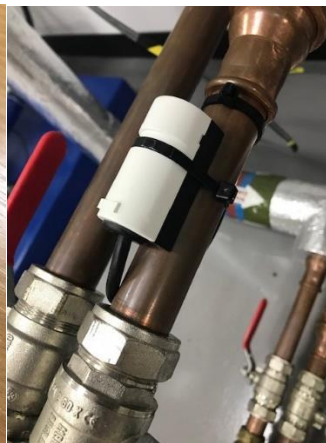
Flow Temperature Sensor on pipework
