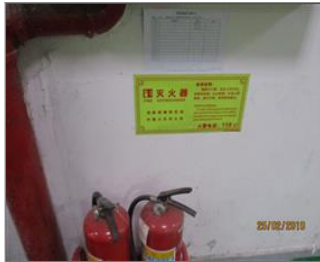
Photo of fire safety equipment Fire extinguisher.jpg
