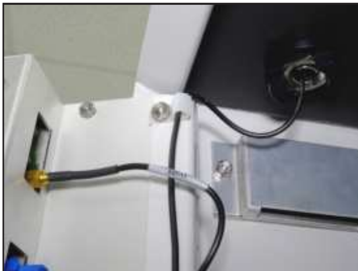
Figure 10. GPS antenna installed and connected.
