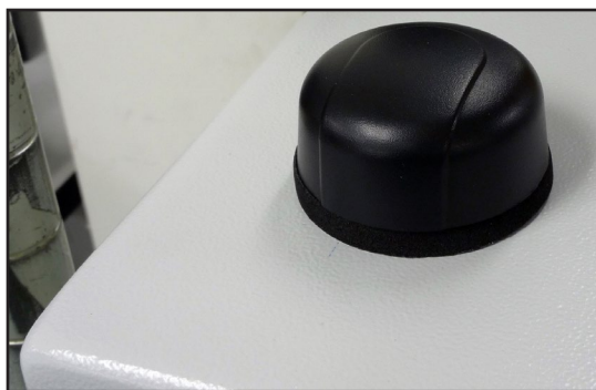
Figure 7. Exterior view of the installed GPS antenna.
