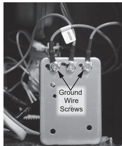
Figure 58 - Location of ground wires
