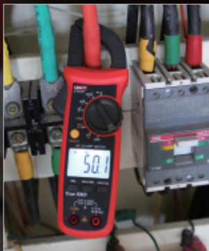
High voltage (600V) frequency measurement
