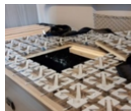
Water Heater Bypass Access
