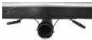
Black/Grey Tank Drain and Valves
