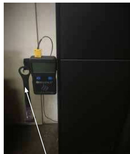
Air and Bypass operating handle/monitor storage.
