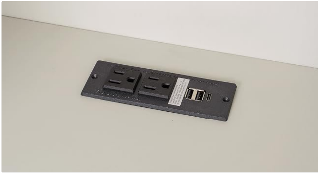
Figure 6: Built-in Power Outlet. Provides convenient charging for devices.
