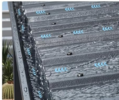
Gutter collects water along the front edge
