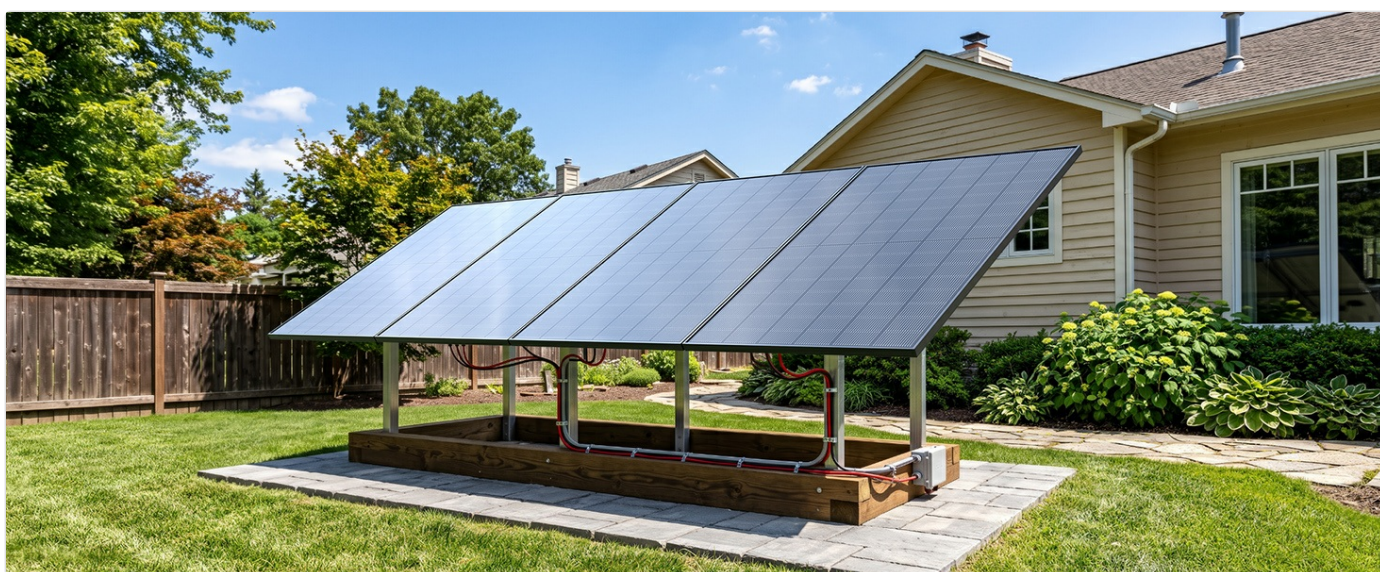
Figure 8: Ground-mounted installation example.
