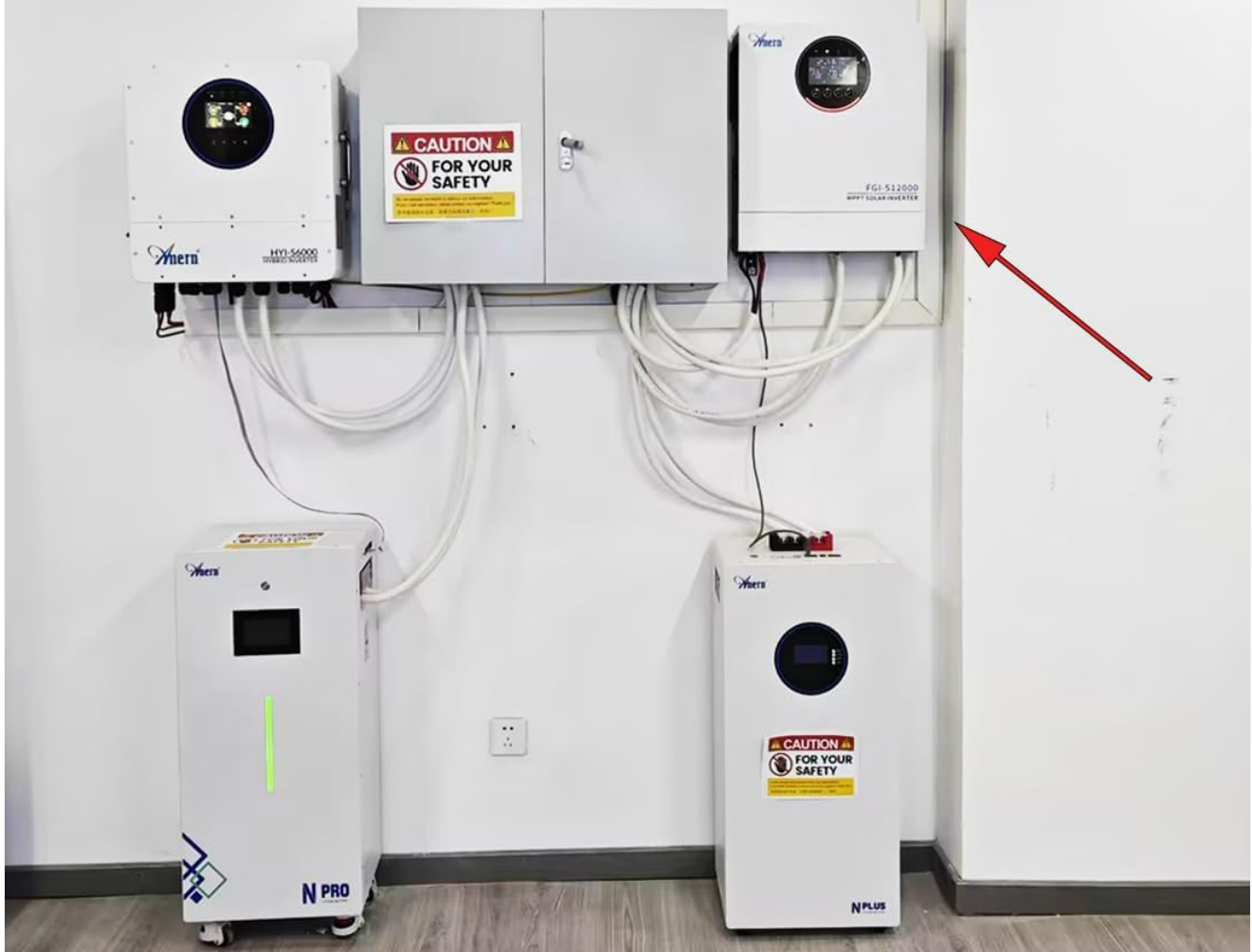
Image 4.3: Application Scenarios. This image displays an example installation of multiple Anern inverters and battery units in a wall-mounted setup, demonstrating a typical application scenario for the hybrid solar inverter system.
