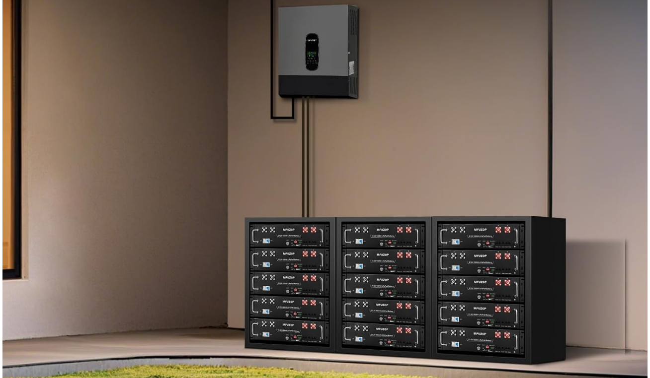
Image 8.1: Multiple MFUZOP 3U rack batteries installed in a rack, demonstrating parallel connection capability for increased energy storage.
