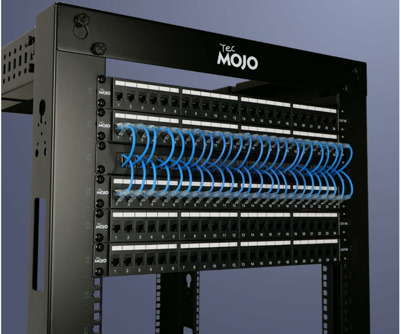
Image: Ultra-slim Tecmojo Cat6a cables organized within a patch panel, illustrating how the design allows for a clean and efficient setup in network racks.
