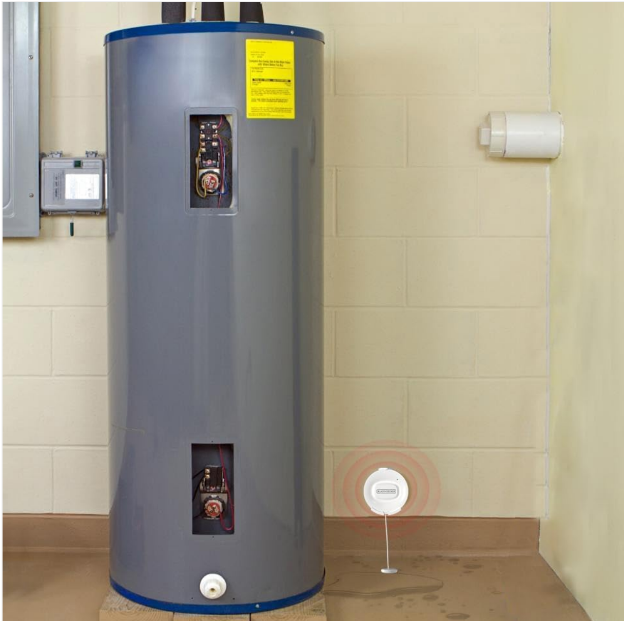
Image 2: Close-up of the water sensor and its probe
