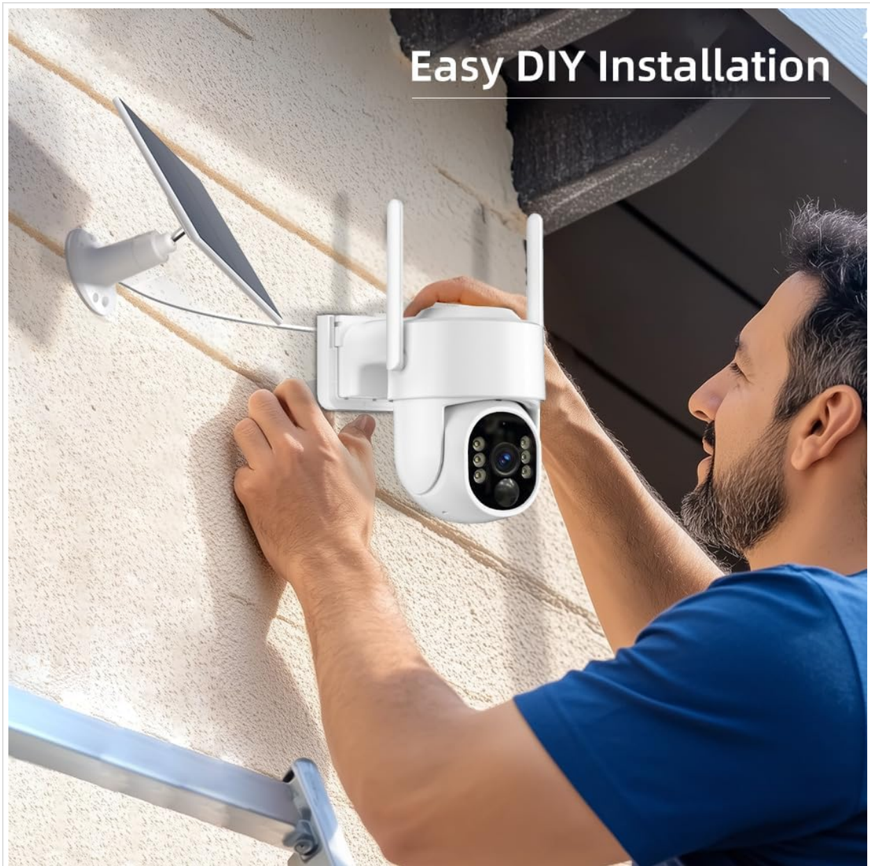
Figure 3: Camera Installation. This image shows a person installing the camera on an exterior wall, demonstrating the ease of DIY installation.
