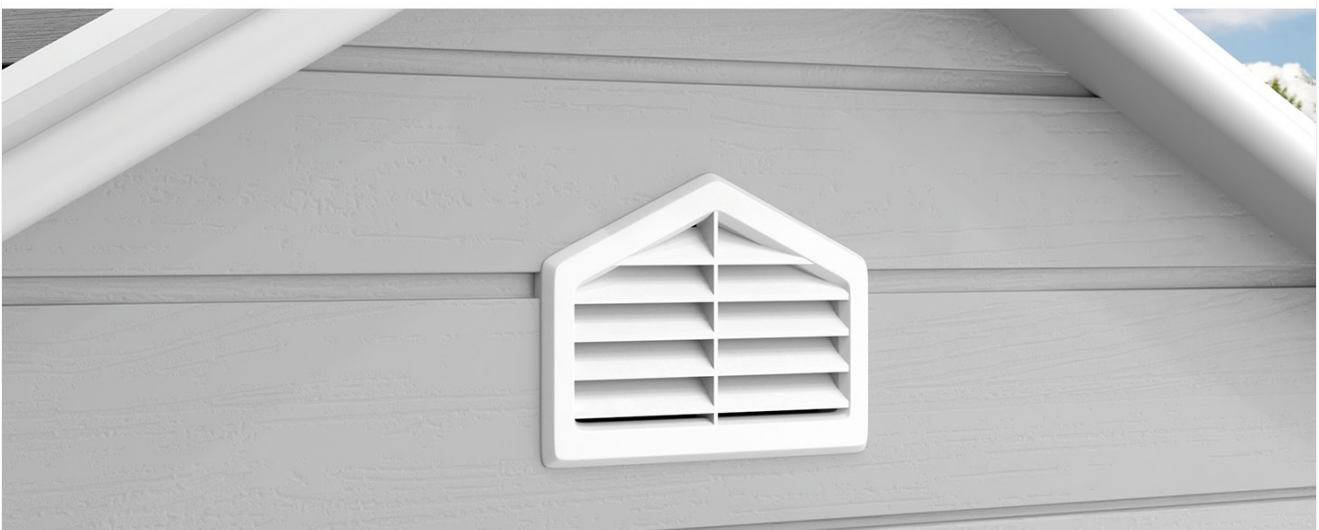
Image 8.1: Air vent for proper circulation.
