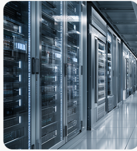
Server Backup Power
